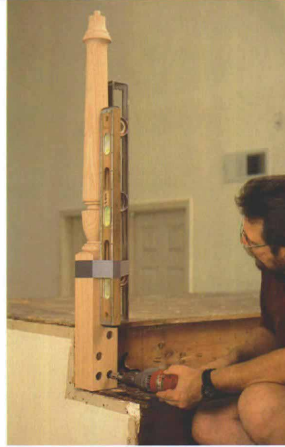
Landing newel is bolted to both riser and tread. Unlike the starting newel, the landing newel is bolted in two directions. The lower left hole provides access to the vertical hanger bolt; lag bolts are driven horizontally into the other three holes.
